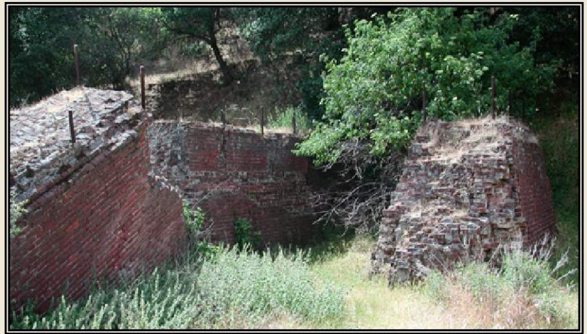
Brick foundation of the hoisting works at the Black Diamond Mine in the Black Diamond Mines Regional Preserve. This is the only structure that remains at Nortonville. The foundation at the left of the photo has cracked in half, and sank into the loose soil where the shaft once was. From the Southport Land and Commercial Company Archives.
